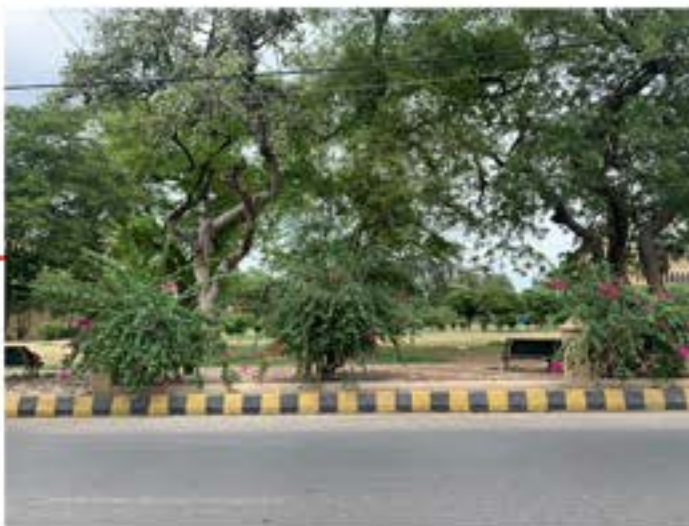
Fence (v) 25' x 0" Missing
