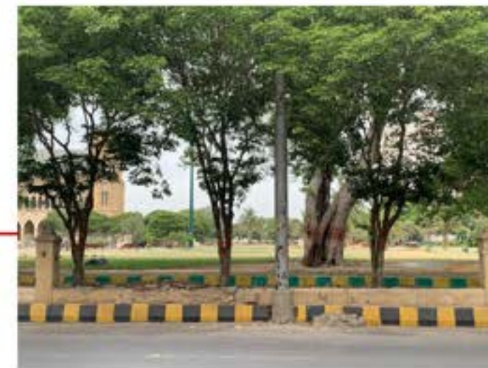
Fence (g) 24' x 10" Missing
