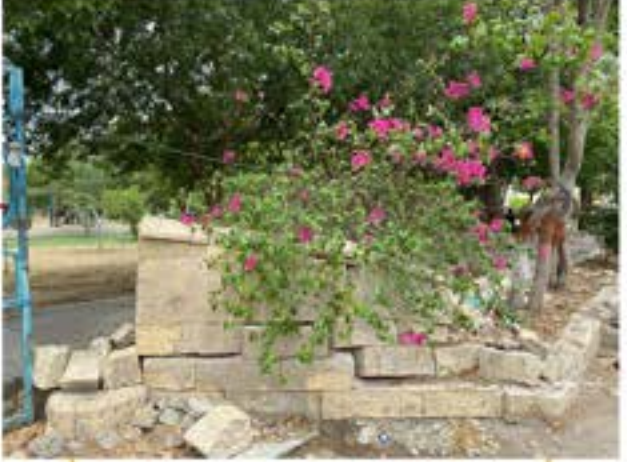
Wall (h) 7' x 3" Damaged
