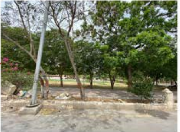
Fence (g) 24' x 2" Missing
