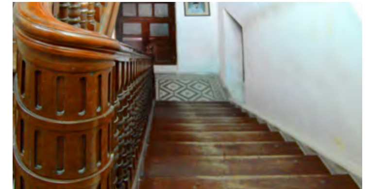
Top: Carved wooden balustrade, wooden staircase / Centre: Gable roof wood truss details / Bottom: Ceramic Floor Image Copyright of Marvi Mazhar and Associates
