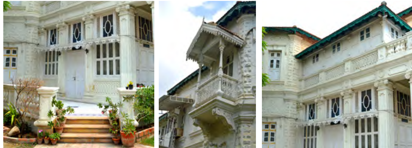
Left: Steps to patio / Centre: West elevation balcony detail / Right: Arched Window with Mouldings Images Copyright of Marvi Mazhar and Associates
