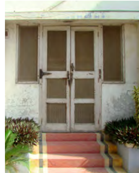
Top Left: Terrazo Steps / Centre Left: Front View / Bottom Left: Details Images Copyright of Marvi Mazhar and Associates
