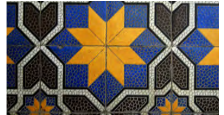
Top: Mosaic tiling / Centre: Tread and Riser Details / Bottom: Jaali Detail-Railing Image Copyright of Marvi Mazhar and Associates
