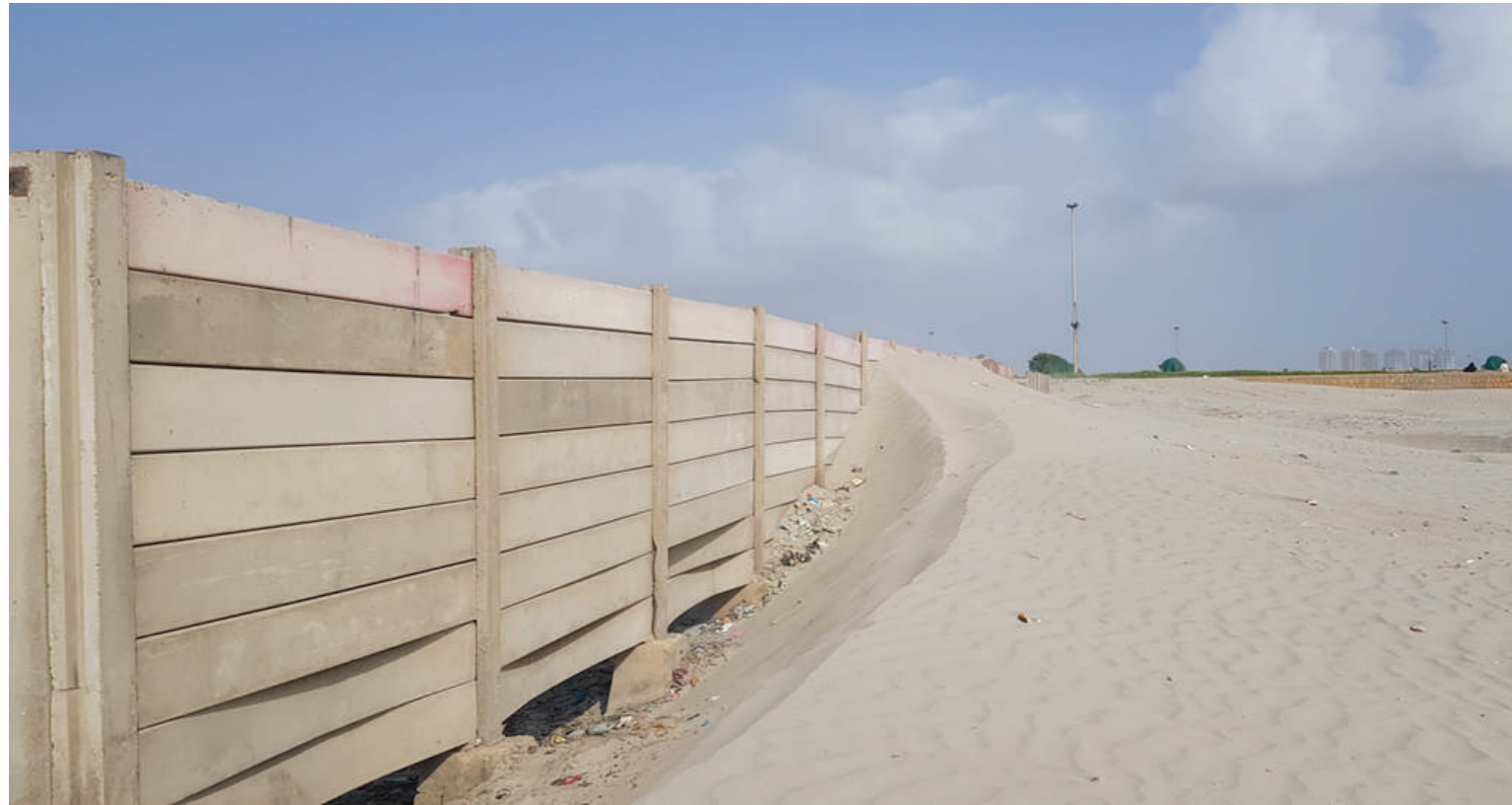
Sand builds up against the wall
