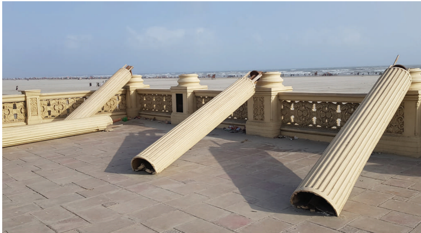
The columns constructed from fibreglass have deteriorated due to the fragility of the structure.
