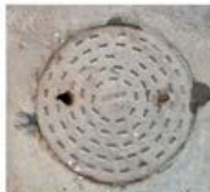
Sewerage Cover Plate
