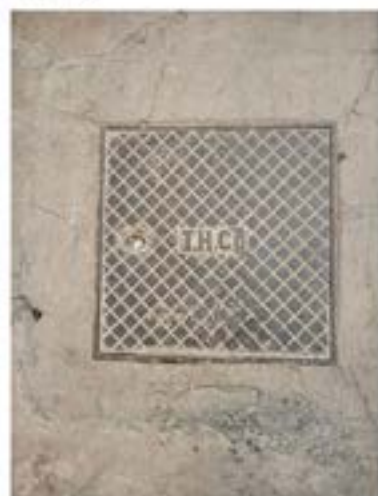
Sewerage Cover Plate
