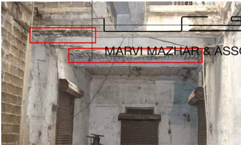
Figure 10-Existing part of the building in dilapidated condition
