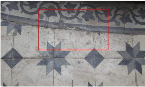
Figure 13-Existing chipped floor tiles
