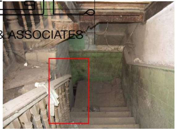
Figure 16-Damaged railings of the existing staircase
