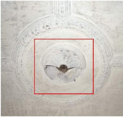
Figure 12-Existing damaged decoration of the ceiling
