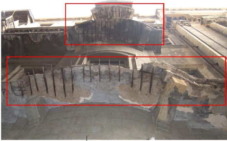
Figure 8-Existing part of the facade in dilapidated condition
