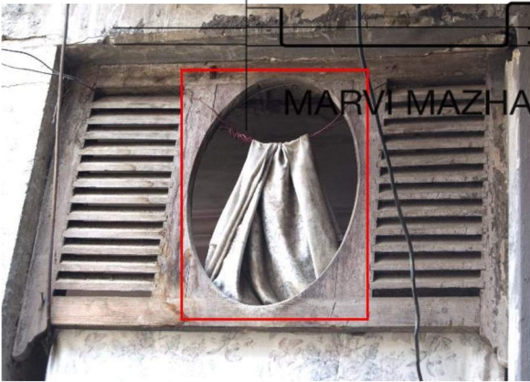
Figure 15-Glass absent in the existing ventilators
